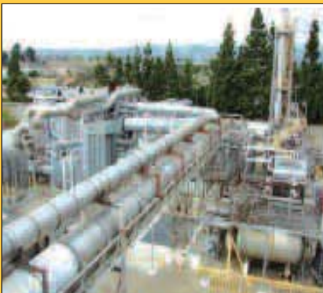
State of the Art Solvent Recovery System
