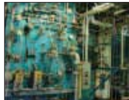
Murray Iron Works Steam Boiler
