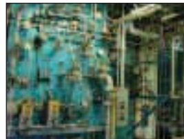
Murray Iron Works Steam Boiler
