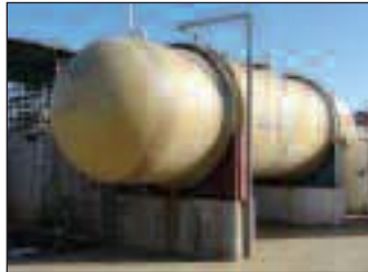
10,000 Gallon Horizontal Fiberglass Tank
