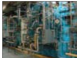
Nebraska Steam Boiler
