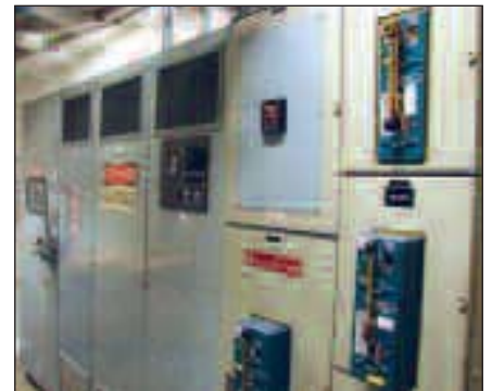
Asco ATS Emergency Switch Control Panel
