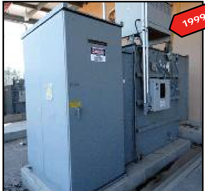
SQUARE D 5000 KVA TRANSFORMER
