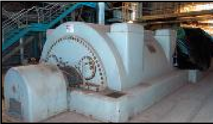
GENERAL ELECTRIC TURBINE/GENERATOR SET
