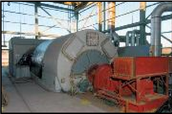
WESTINGHOUSE TURBINE/GENERATOR SET
