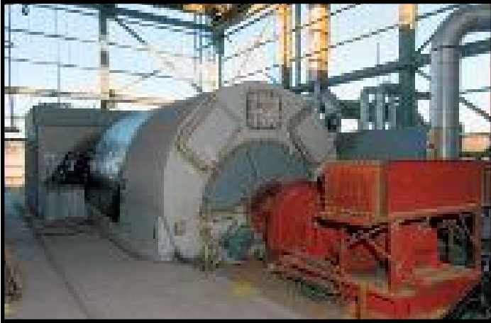
WESTINGHOUSE TURBINE/GENERATOR SET
