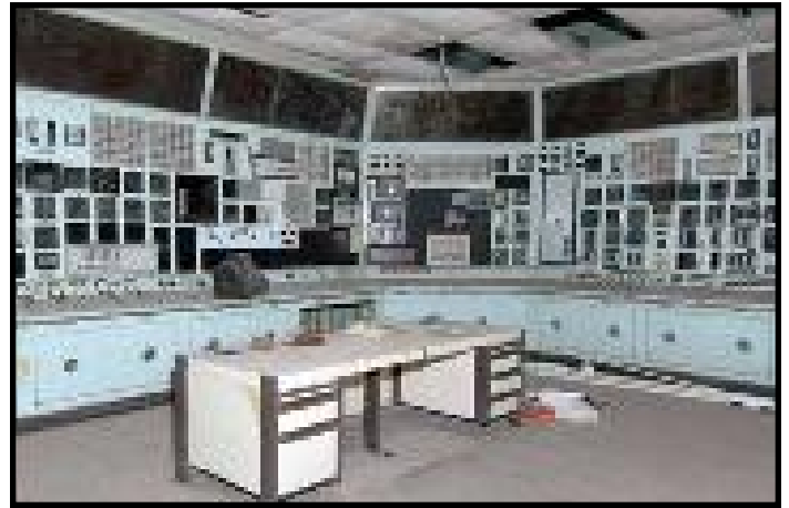
GENERATOR CONTROL ROOM
