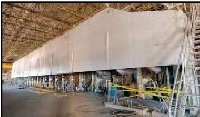
DOMINION PAPER MACHINE DRYER SECTION
