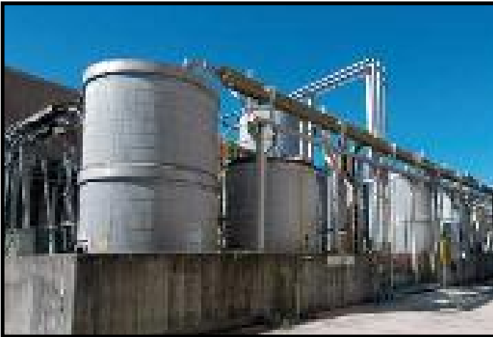
JACKETED TANK FARM
