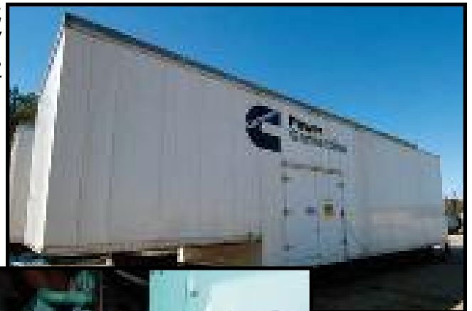
> ONAN 2000KW DIESEL GENERATOR SET
