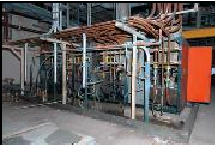
HIGH VOLUME HYDRAULIC SYSTEM
