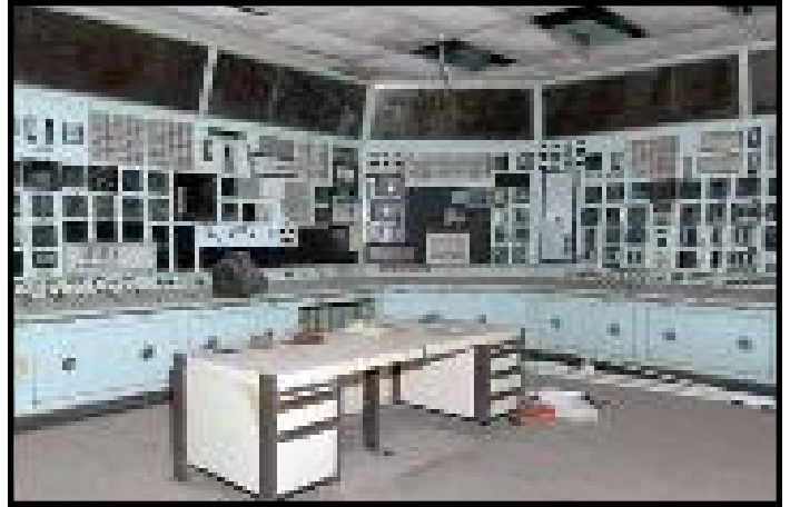
GENERATOR CONTROL ROOM
