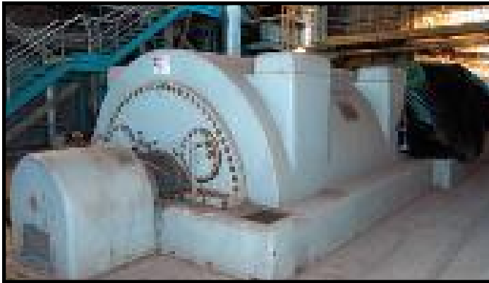
GENERAL ELECTRIC TURBINE/GENERATOR SET
