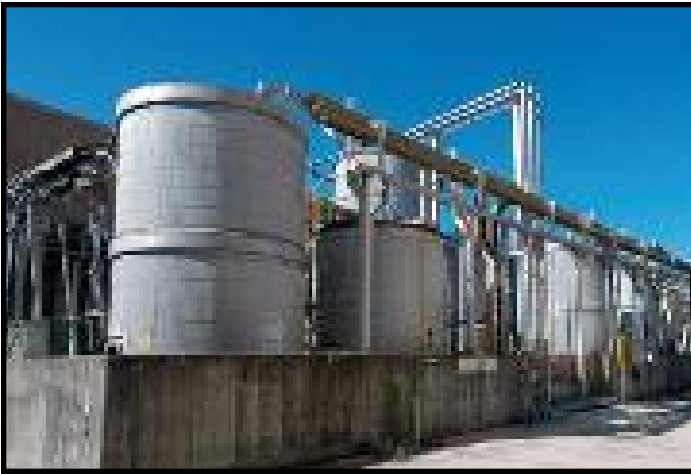
JACKETED TANK FARM
