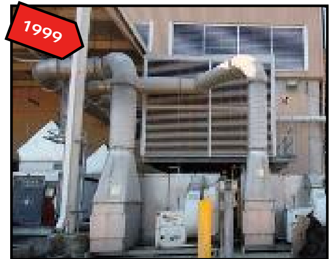
MARLEY COOLING TOWER SYSTEM
