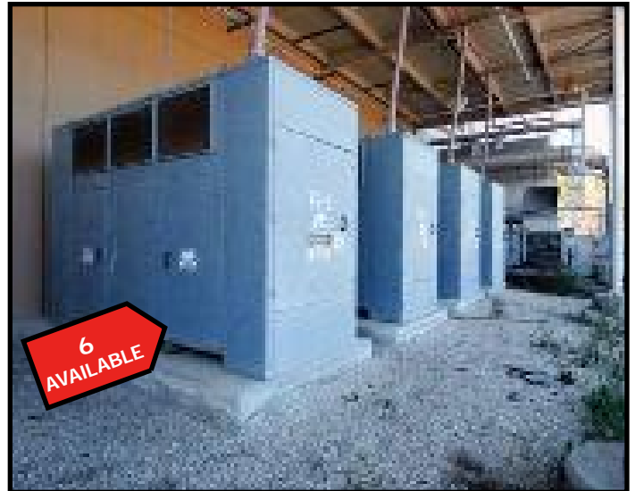
SQUARE D, 3000 KVA TRANSFORMERS
