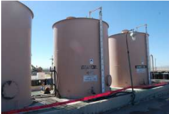
Inv# 109 (2) Steel Tanks - Approx 45' Diameter x 45' Height
