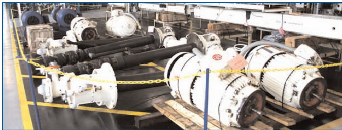
VIEW OF HELLER LINE COOLANT PUMPS & MOTORS
